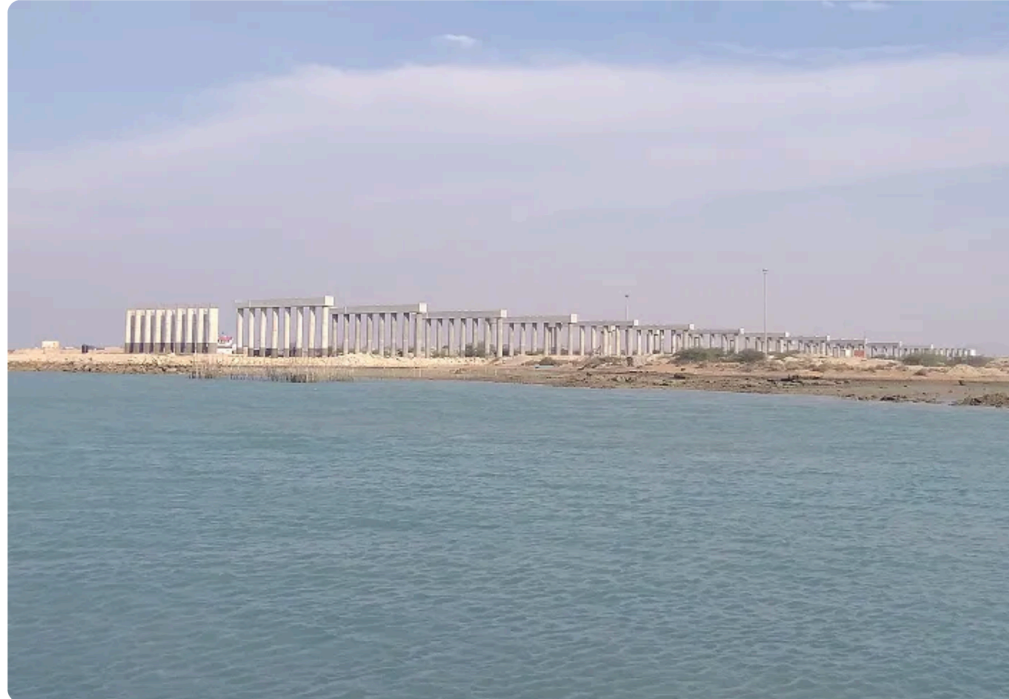
The Persian Gulf Bridge, with its massive foundations and caissons, is under construction [File: Courtesy of Creative Commons]
